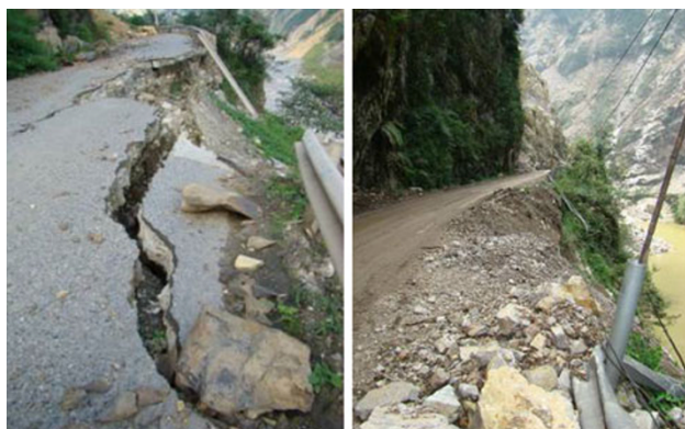
Fig. 1 Embankment slope landslide in Wenchuan earthquake
