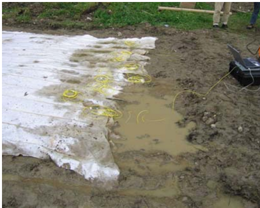
Fig. 13 Sensor-based geotextile mat being installed during construction of a gravity dam in Solina/Poland (textile: Saxon Textile Research Institute (STFI) e.V. Chemnitz).
