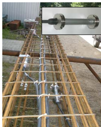
Fig. 4 Sensors fixed at the cage of reinforcement for a 19-m-length concrete pile (above right: sensor body).
