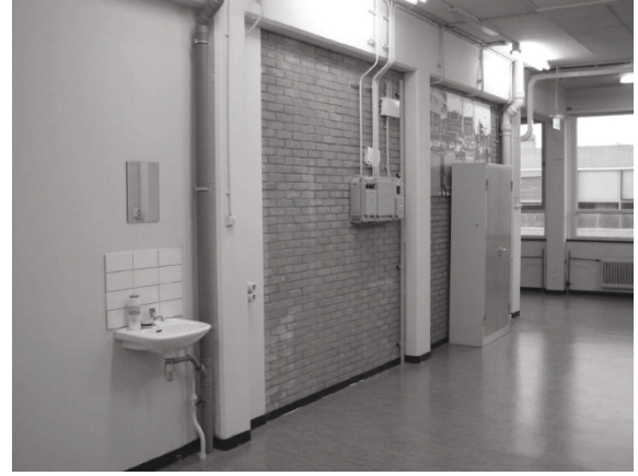
FIGURE 1: Photograph of the corridor wall.
