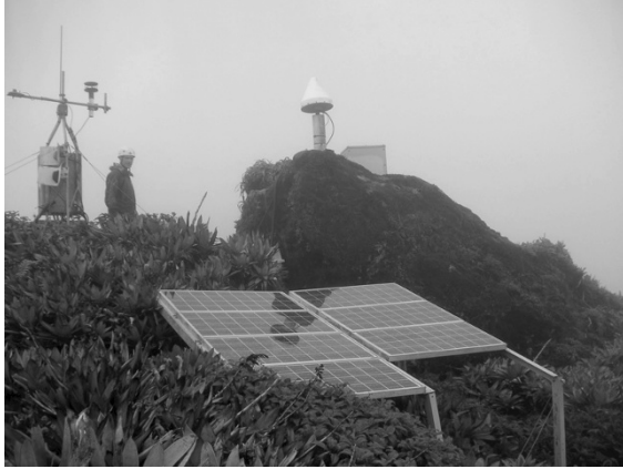
Fig. 5. Example of power and transmission equipment for the permanent station Sanner operating at the summit of La Soufrière in Guadeloupe. The solar panels have a nominal power of 378 W for a power consumption of 20 W. The buffer accumulators have a capacity of 300 A h. No power failure has ever occurred at this station during 8 years of continuous operation.
