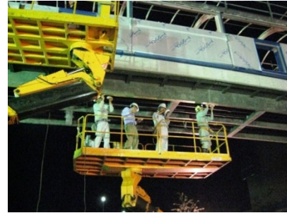
Fig. 13 Optical fiber sensor installation on girder.
