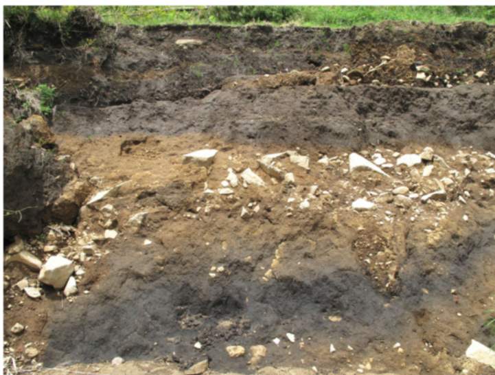
Fig. 9 Soft volcanic ash soil with gravel around the Aso Bridge landslide
