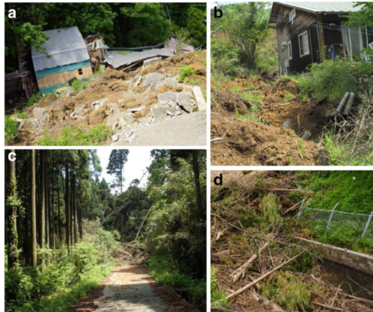
Fig. 3 Damages caused by earthquake-triggered landslides in Kumamoto; a collapsed houses, b broken underground pipelines, c road destroyed by the landslide mass, d damaged water channel
