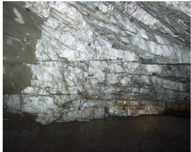
Fig. 1 Slabbing failure in the roof of a 3-year-old mine drift excavated in quartzite at 1,000 m depth. The roof was exposed when another parallel drift was excavated
