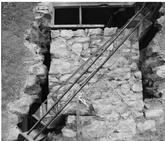
Fig. 9. Un-reinforced panel tested at Colle Umberto.
