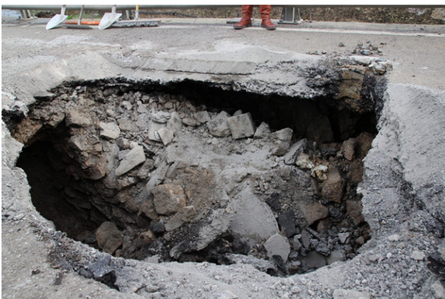
Fig. 7. Photo of the cavity below the PR26C detected by the GB-InSAR on 4 February 2014.
