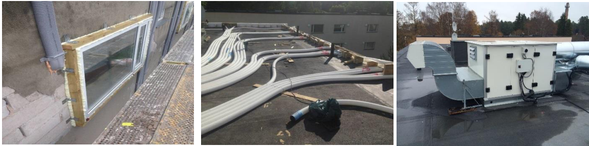
Fig 6. Ventilation ducts in the façade insulation (left), ventilation ducts in the roof insulation (centre), and a central AHU on the roof (right).
