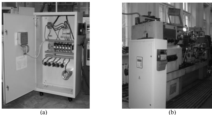
Fig.3. Automatic Reactive Power Control and Compensation devices ARPCC: (a). general view of ARPCC; (b). ARPCC connected to lathe 16K20
