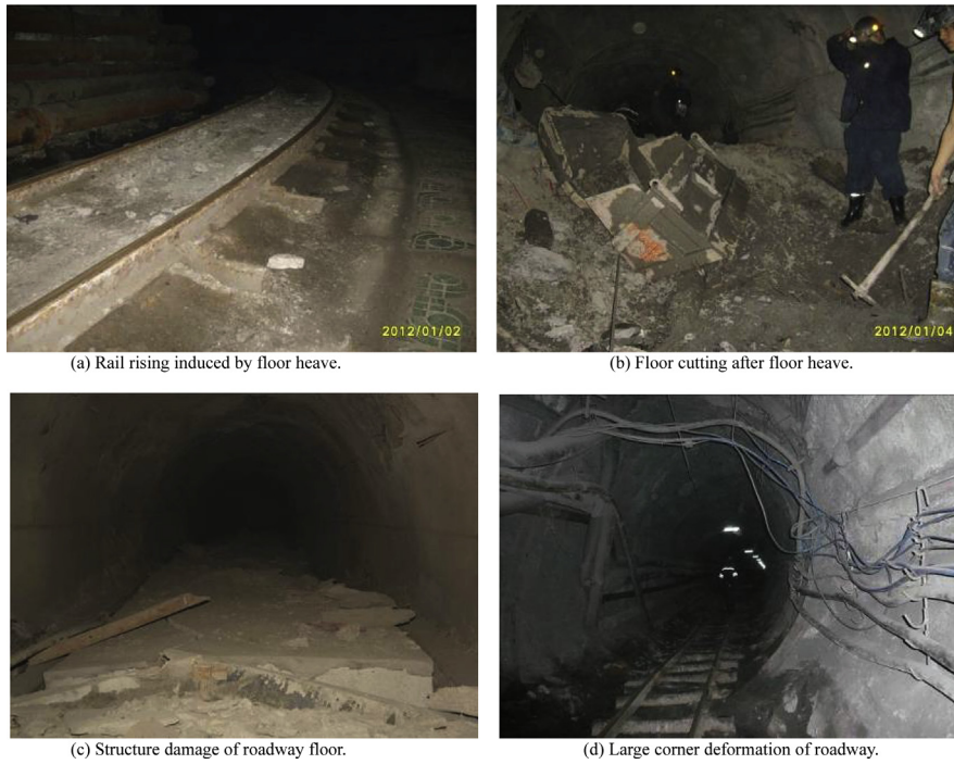
Fig. 3. Deformations of roadway floor.
