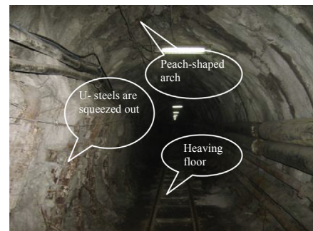
(a) Two sidewalls are squeezed, which is caused by large horizontal stress, forming a sharp peach-shaped roadway and serious floor heave.
