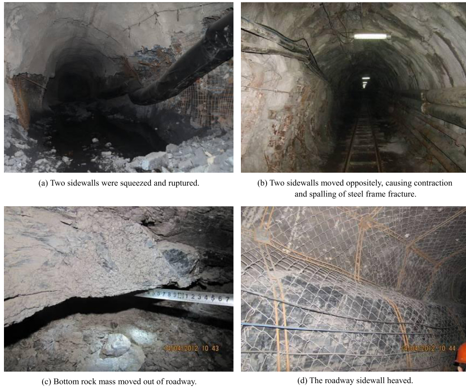
Fig. 1. Deformations of sidewalls of a roadway.
