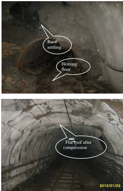
(a) Large convergence of roof and floor caused by vertical stress.
