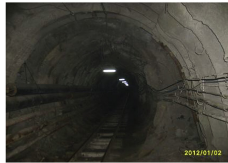
(a) The horizontal and vertical directions are in high stress level, and the whole section shrinks.
