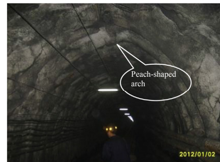
(b) Two sidewalls are squeezed, which is caused by large horizontal stress, forming a sharp peach-shaped roadway.
