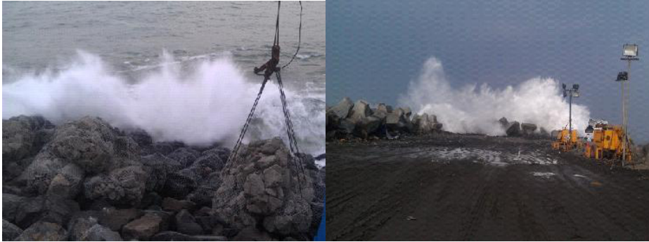
Fig. 7. The measure combining wire mesh gabions with artificial armours for breakwater head protection during construction period
