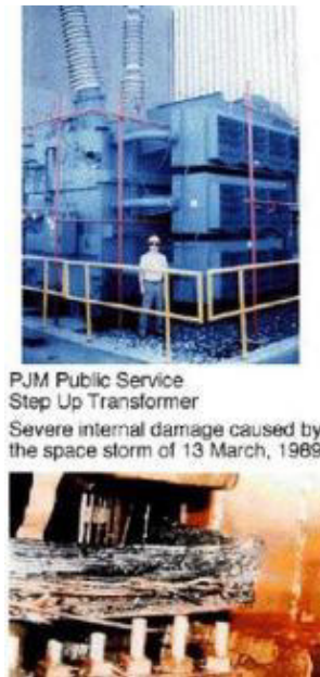
Fig.4. Burned Transformer in Hydro-Québec's power grid in 1989 (Schoch R. M., 2012)
