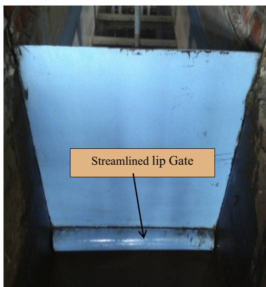
Figure 1 Streamlined lip gate in flume.
