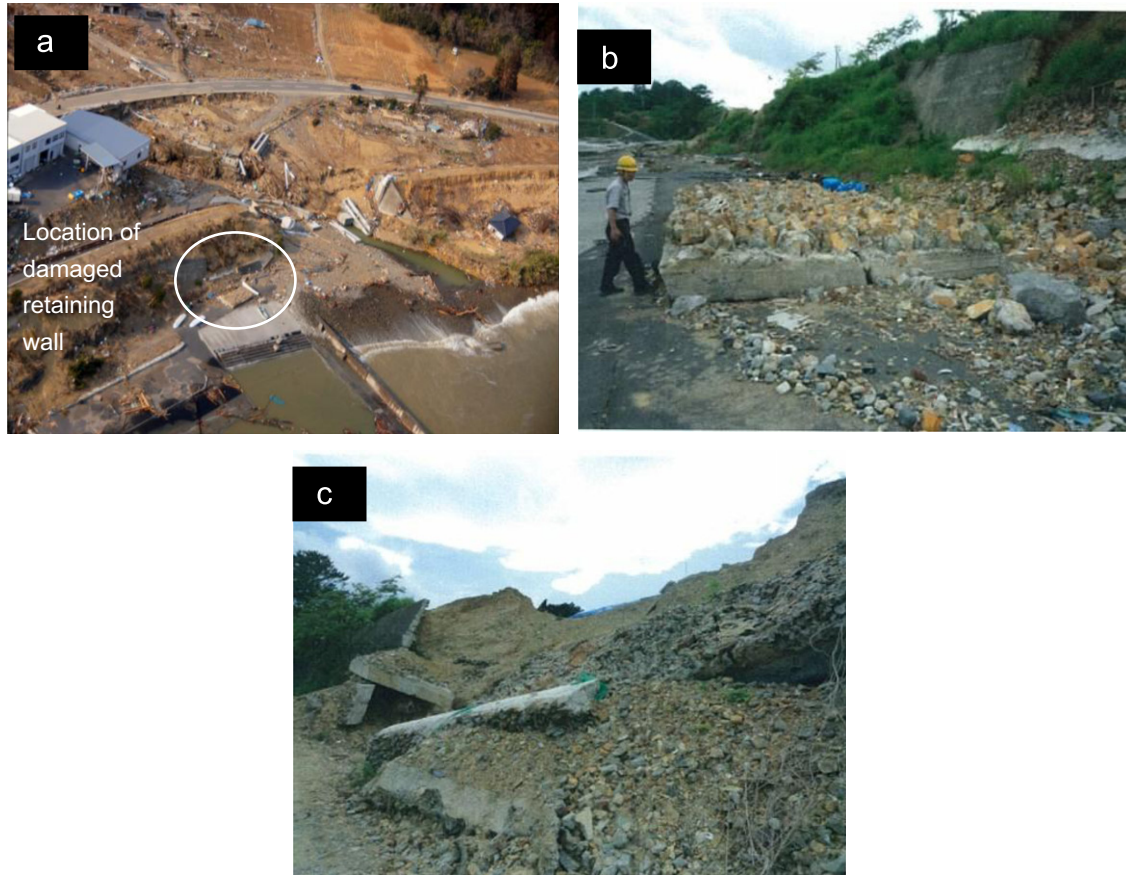
Fig. 19. (a), (b) and (c) Tsunami-induced damage to retaining wall beside Ohsawa-gawa bridge along JR Kesennuma line at 54k098m between Motoyoshi and Koganezawa stations.
