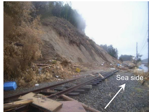
Fig. 6. Tsunami-induced damage to cut slope along JR Ofunato line at 89k900m between Wakinosawa and Otomo stations.
