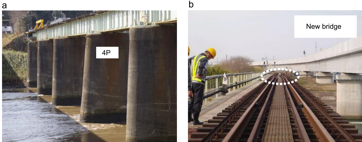
Fig. 13. (a) Inclinometer and settlement of Pier no. 4 of Naka-gawa bridge along JR Suigin line at 0k956m between Mito and Hitachi-aoyagi stations and (b) rail track deformation on the bridge.
