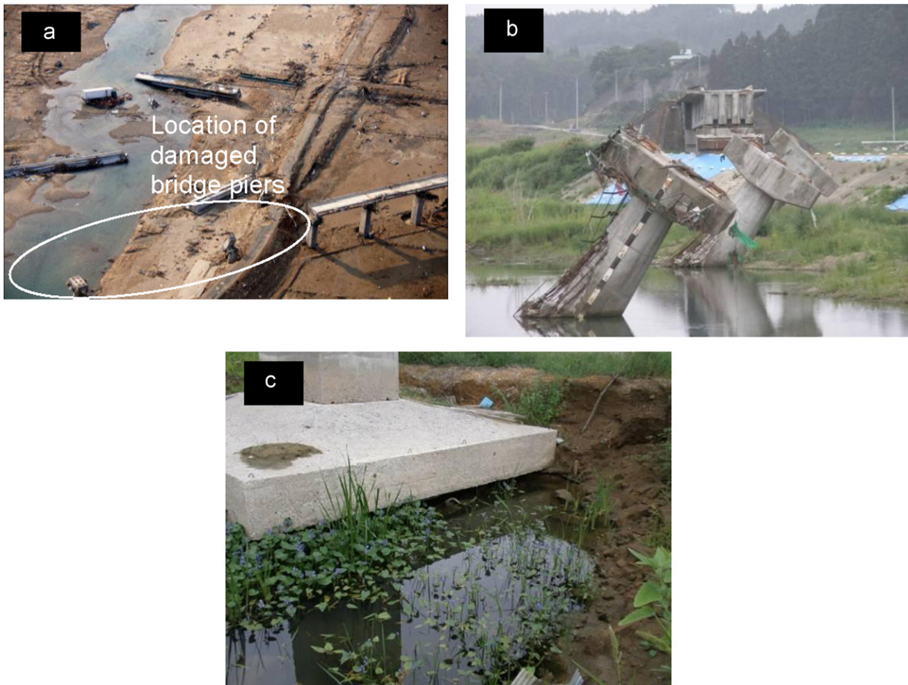
Fig. 21. (a), (b) and (c) Tsunami-induced damage to Tsuya-gawa bridge on JR East Kesenuma line at 50k099m between Rikuzenkoizumi and Motoyoshi stations.
