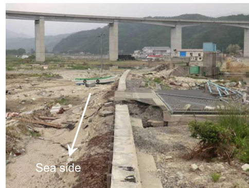
Fig. 8. Tsunami-induced damage to Orikasa station on embankment along JR Yamada line.
