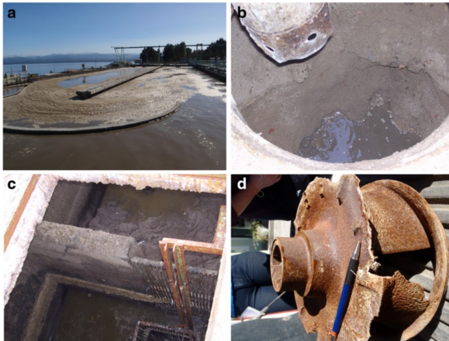
Fig. 11 Bariloche wastewater treatment system a biological reactor showing some Nocardial foaming; b and c sewer lines and junctions inundated with ash; d ash-accelerated pitting and thinning damage to sewage pump impeller
