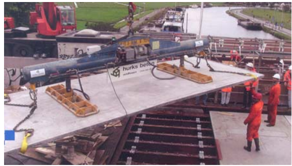
Fig. 3 Assembly of precast deck panels in reinforced ultra high strength fiber reinforced concrete (Kaag Bridges, The Netherlands)
