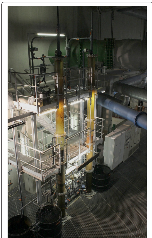
Figure 3 Dual-media rapid filters of the pilot plant in the PEP Tegel in Berlin.
