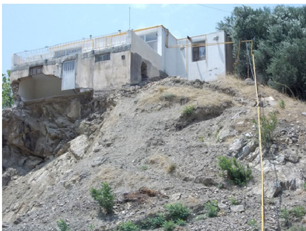
Fig. 3 A house in Rudbar. The front part of the house was still in ruins in 2012 and the back part of the house was reconstructed and built over many years after the 1990 Rudbar earthquake. Note the unsafe connection of the house to gas ( yellow pipe at the right side of the photo). Photograph by M. Ibrion, 2012
