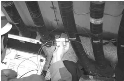
Fig. 10 Current monitoring of a 6.6-kV power cable using a reflection type sensor.
