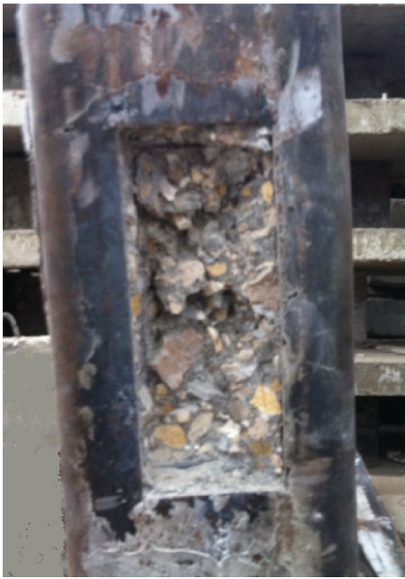
Fig. 11 Typical mode of failure for strengthened RC column using steel angles and strips
