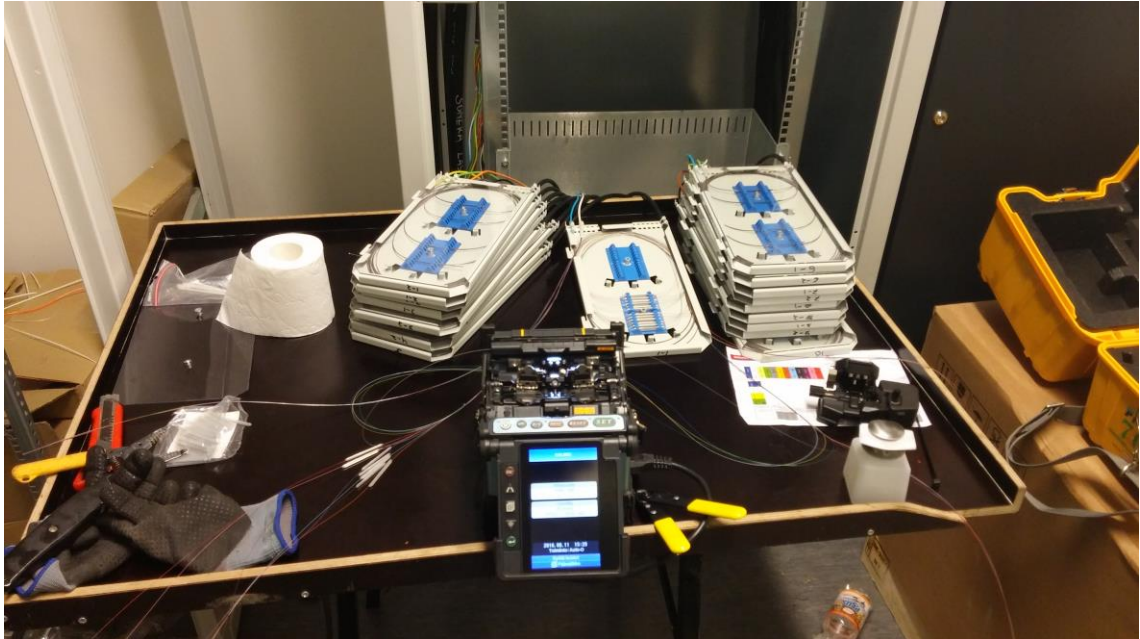
Figure 10. Optical fiber splicing equipment and Fusion Splicer.
