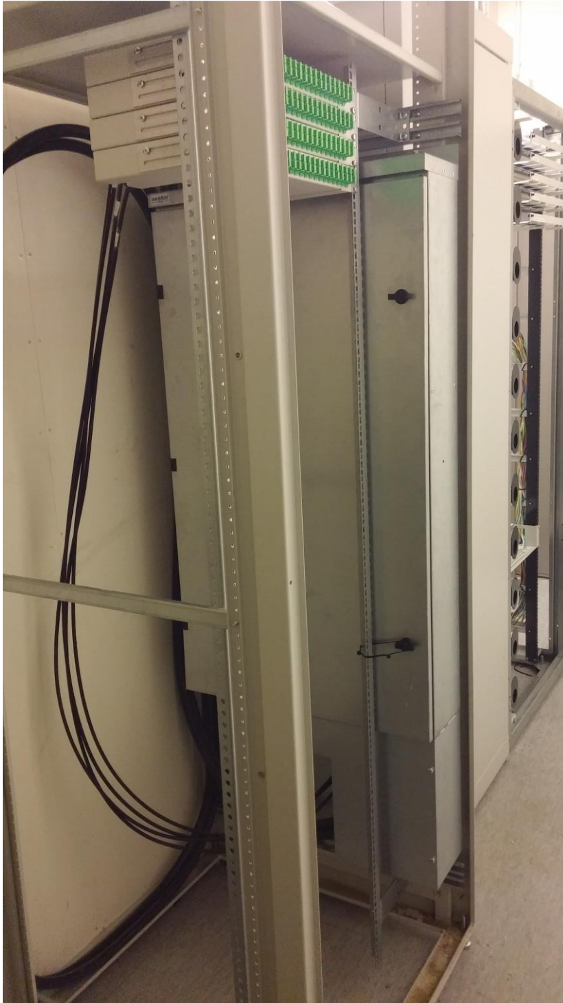
Figure 16. 864 panel rack and splicing cabin.
