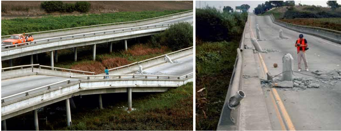
Figure 1: Failure of the Struve Slough Bridge due to Loma Prieta Earthquake, USA [18].
