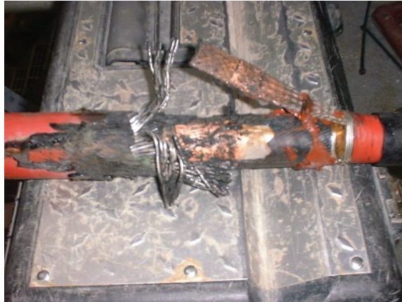
Fig. 4.26. A damaged MV cable joint [108].
