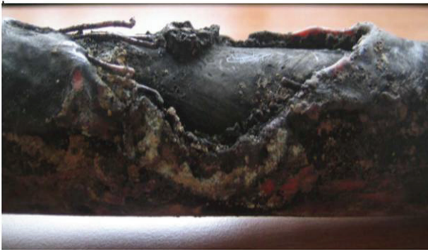
Fig. 4.27. A damaged part of the XLPE cable [109].
