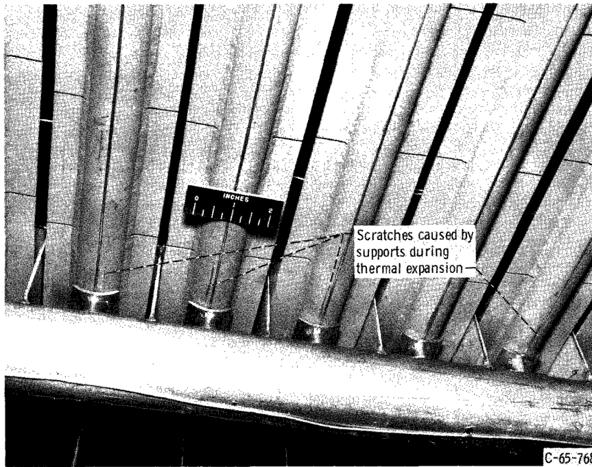
Figure 7. - Outlet-end oil-cooled support showing tube mounting. Relative motion during operation is indicated by scratches near bottom of tubes.
