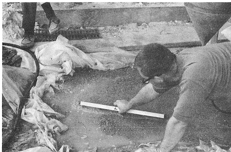
Fig. 7 Leveling Soil Surface While Conducting Field Tests on Saturated Colorado River Sand
