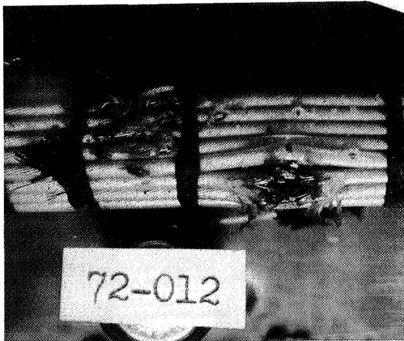
Figure 12. Typical damage to cable type 1.
