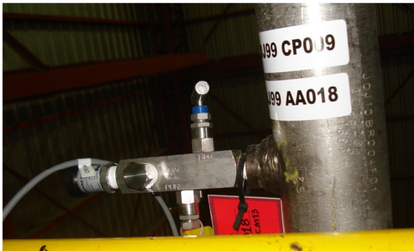
Figure 8. Pressure transmitter installed on piping upstream of one air valve.
