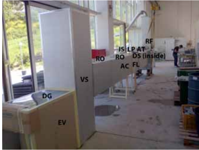
Fig. (4). Dust ventilation duct with measuring instruments.
