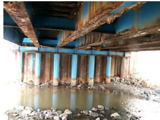
Figure 2. Corroded steel bridge girders (Photo courtesy of Termarust Tech) [4]
