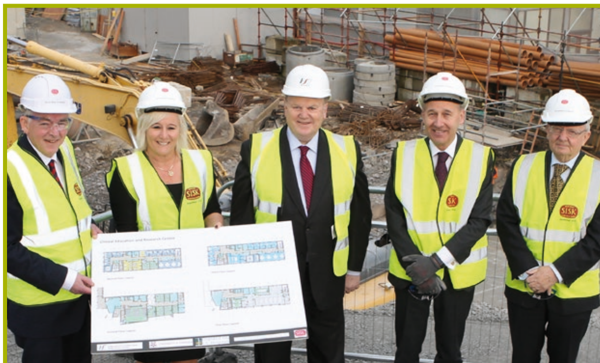
▲ Inspecting building works at the Clinical Education and Research Centre, University Hospital Limerick were (L-R): Prof. Don Barry, President, University of Limerick; Prof. Colette Cowan, CEO, UL Hospitals; Minister for Finance, Michael Noonan TD; Prof. Michael Larvin, Head of UL's Graduate Entry Medical School; and Prof. Niall O'Higgins, Chairman, UL Hospitals
