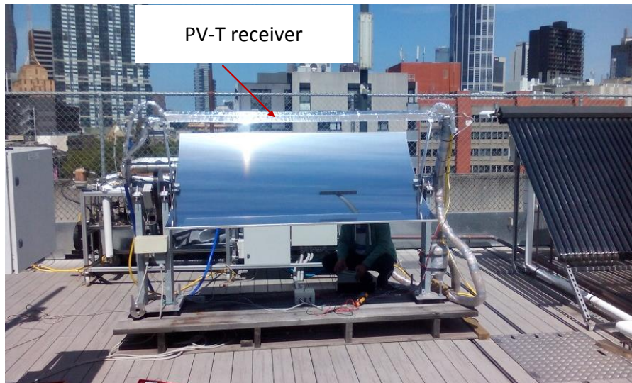
Fig. 6.11 The receiver-trough combination at the roof of RMIT University
