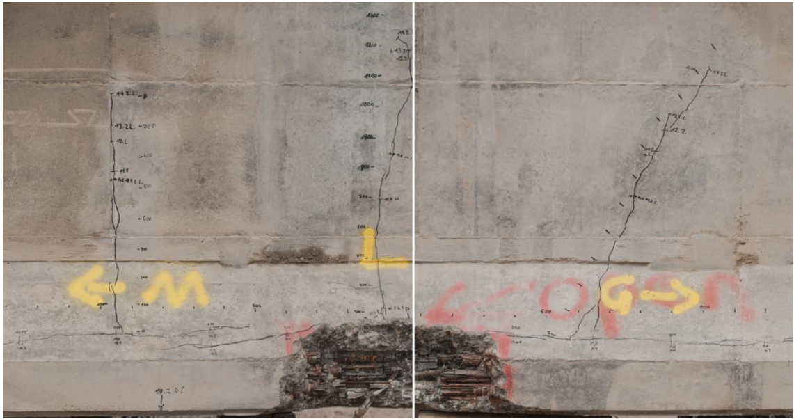
Figure 7: Cracks observed in damage scenario #4
