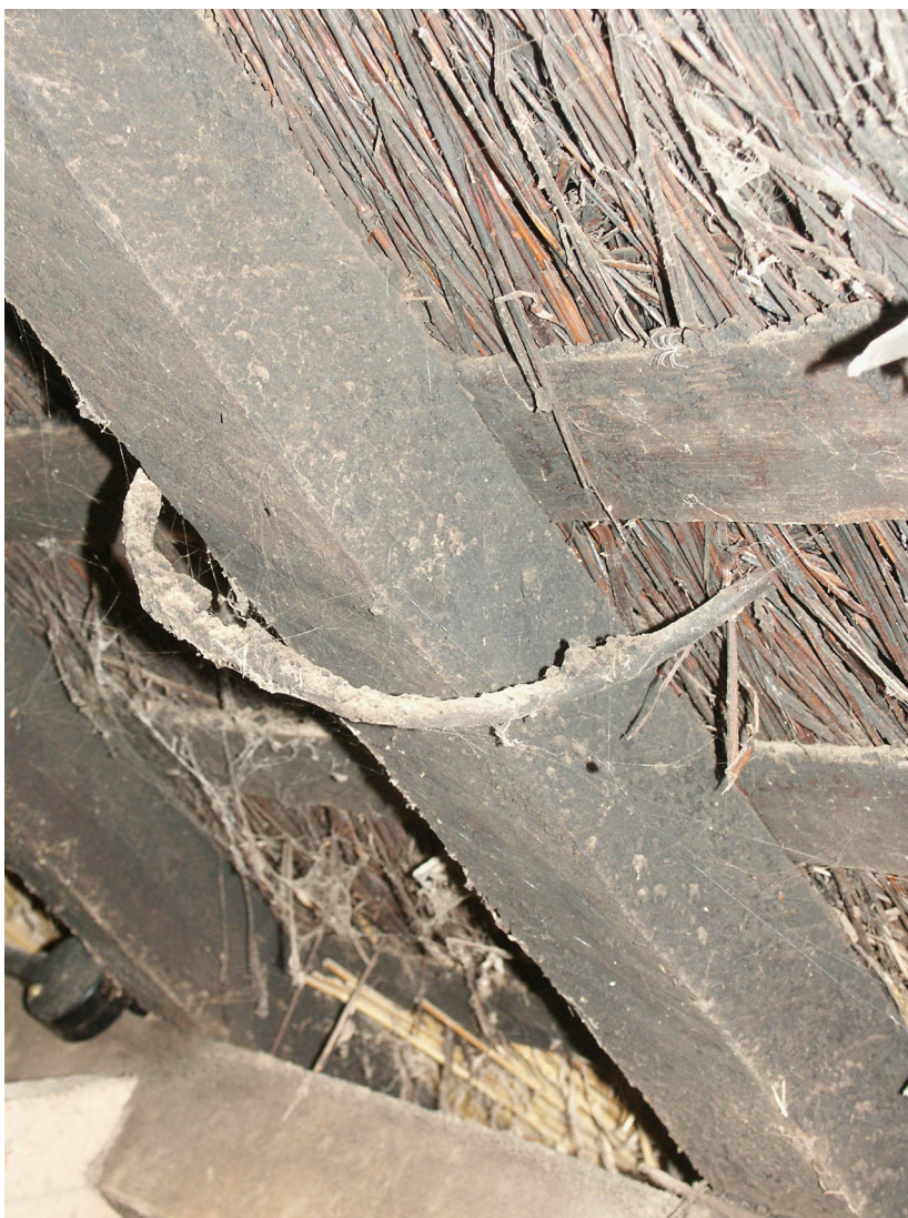
Fig. 18. Elley, Colebrooke, Devon (cf. Fig. 5): The interior of the roof, showing the rafters, thatch, lath and tie (NWA).
