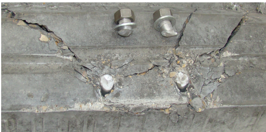
Figure 8. Combination of a concrete cone failure and the connector fracture
