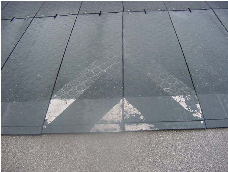
Figure 24. Pavement Markings After Approximately Six Months
