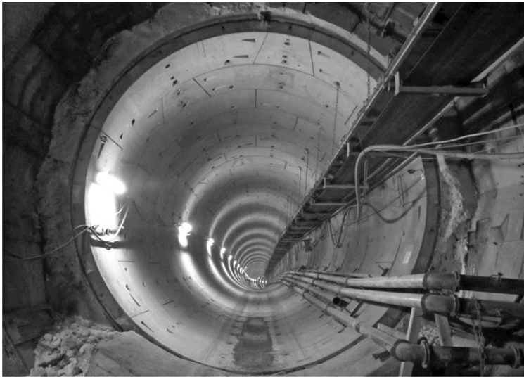
Fig. 3. View of the hardened grout as can be seen in the enlargement for a station in Prague Metro (photos Mapei's archive).
