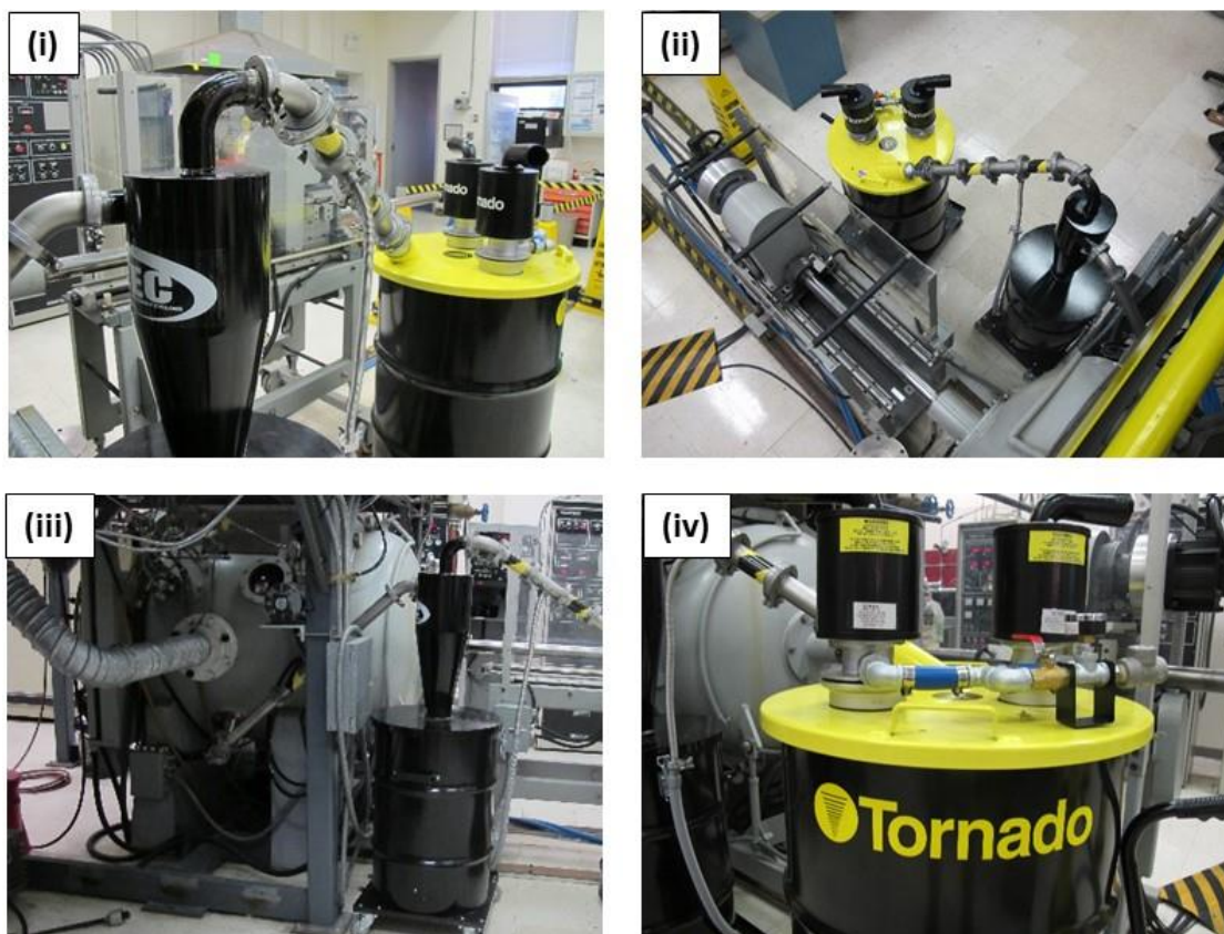
Figure 24. Ruwac cyclone and Tornado pneumatic vacuum system connected in series for dry collection at room temperature: (i) side view of setup; (ii) overhead view of setup; (iii) exhaust exits chamber and enters cyclone; and (iv) exhaust exits cyclone and enters twin pneumatic suction pumps.
