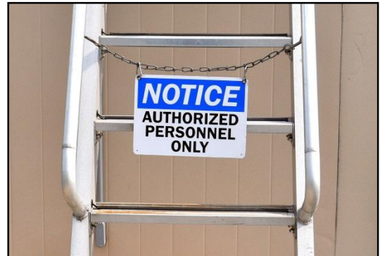
Figure 3-4: Notice on stairway access to roof
