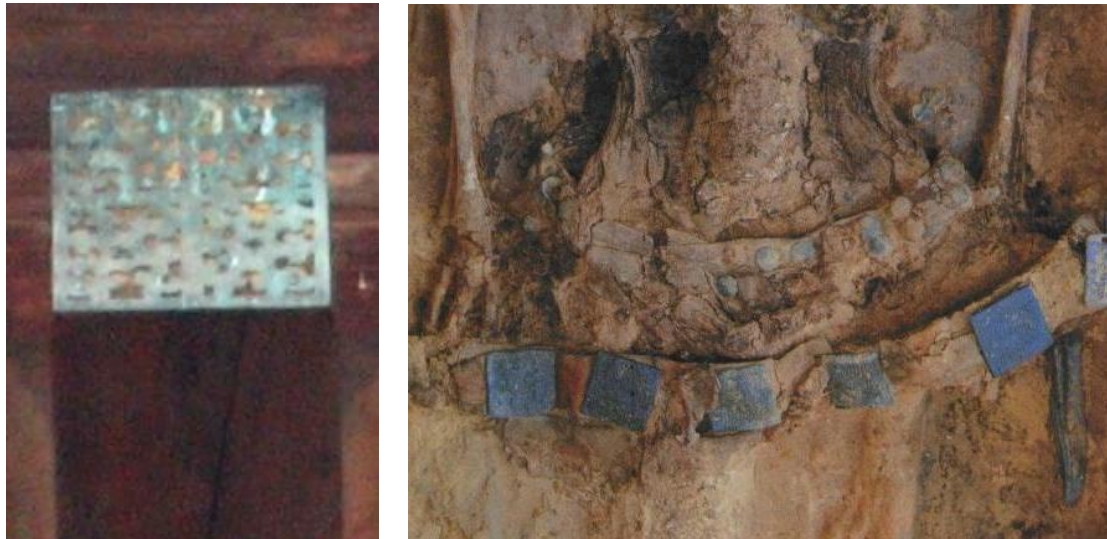
Figure 5.28 (Left:) Metal openwork plaques protecting the exposed ends of the cantilever arms supporting the roof eaves of the Seven Story Pagoda at Horyūji (photo by author)
