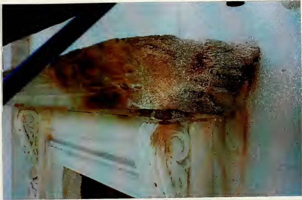
Figure 3.13: A Sheffield window header that had been covered with bituminous bird-proofing. The corner shows the effects of trapped moisture. This part of the stone could be removed merely by scraping the surface.
