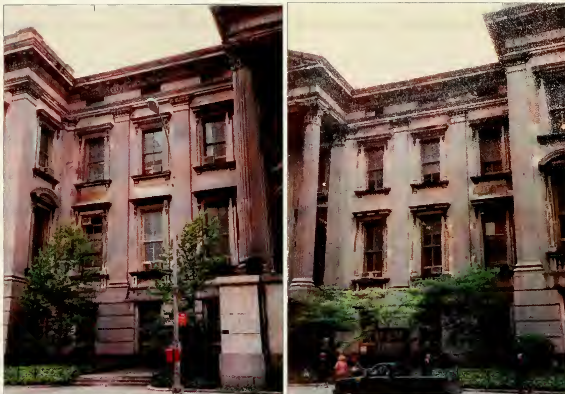
Figures 3.1 & 3.2: Discoloration on the north façade, east and west sides of the portico. May, 1989.
