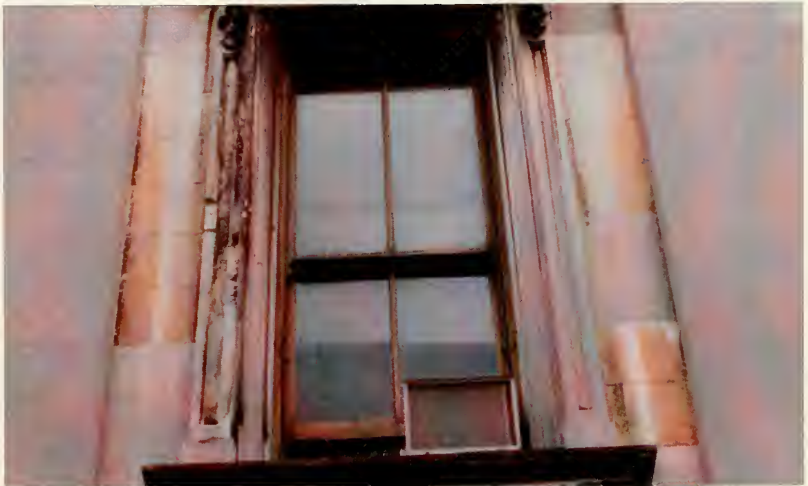
Figure 3.10: Iron-stained marble, probably Sheffield, interspersed with blocks of Tuckahoe. Iron staining may be due to the leaching out of ferruginous minerals such as pyrite. Note how the stone has been washed white in areas of rain runoff near the Tuckahoe marble while the Tuckahoe has remained a solid gray color. Photo taken May, 1989.
