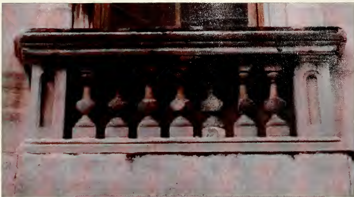
Figure 3.5: Tuckahoe marble balusters showing extreme degradation due to weathering. Characteristic gray discoloration and blackening from the accretion of pollutants are evident. Projecting elements of both types of marble tend to look alike because of pollution staining. Photo taken May, 1989.
