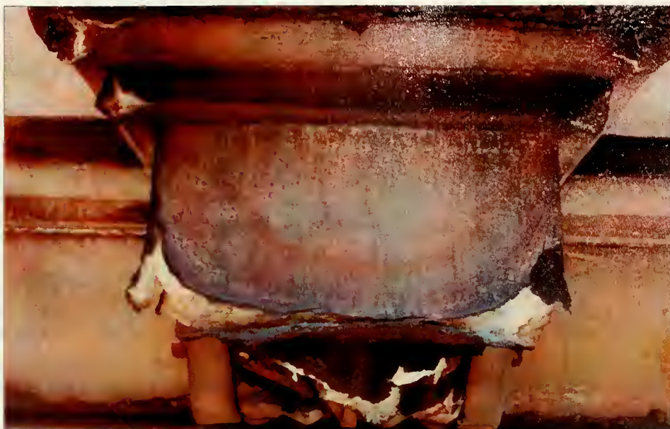
Figure 3.17: A modillion appears to be splitting at the seams due to continued freeze/thaw cycling beneath a hard surface crust of gypsum. Note the semicircular patterns of brownish and blackish iron deposits due to the diffusion of iron leachates and other atmospheric pollutants.
