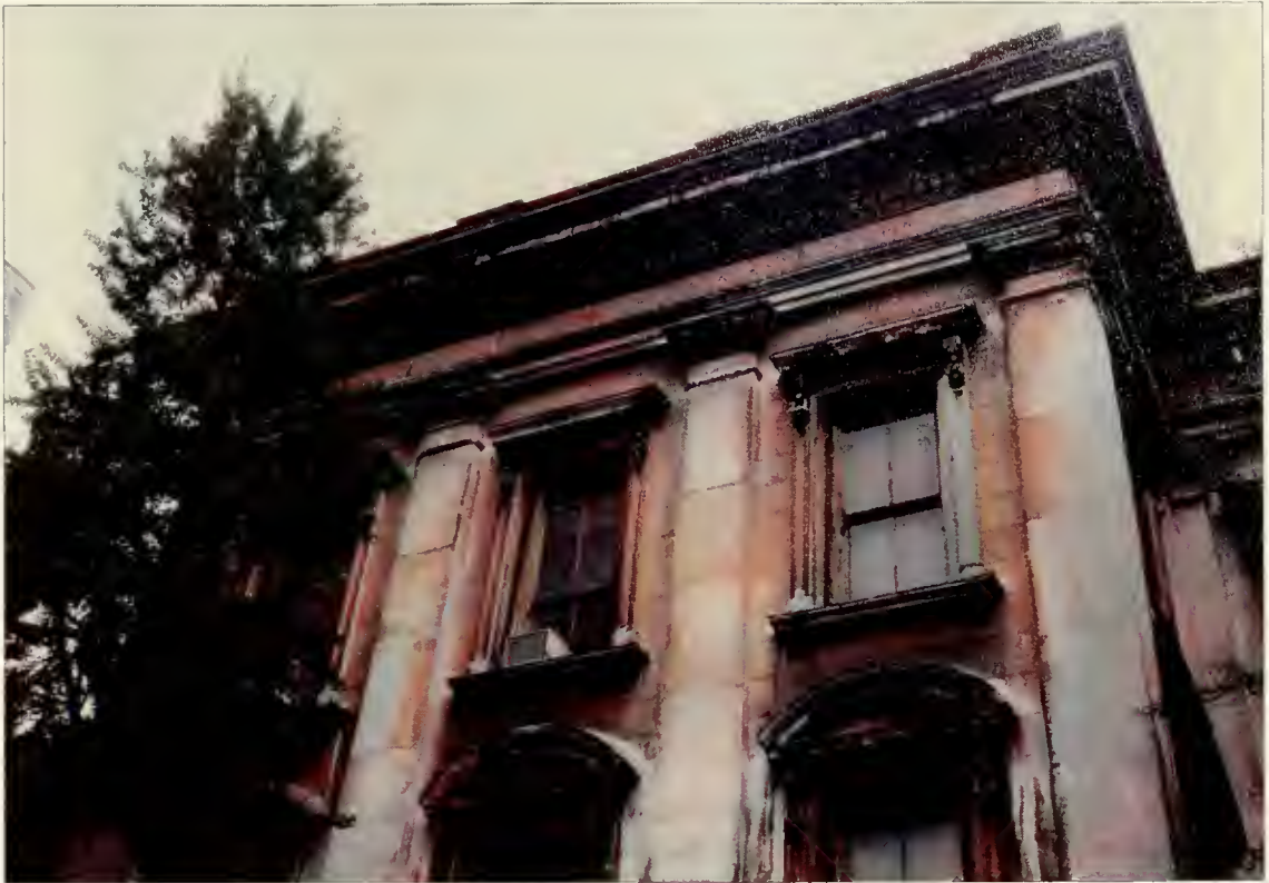
Figure 3.11: South facade, west end, May, 1989. Extreme staining is visible across the entire surface. This type of discoloration is typical of Lee marble, a stone quarried within 20 miles of Sheffield, MA. The south façade exhibits the worst weathering on the building.
