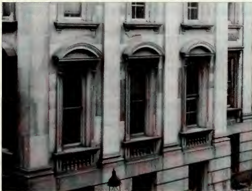
Figure 2.5: Close-up view of the same photograph showing differential staining of exterior marble around the second floor windows. The darker blocks are probably Sheffield marble.
