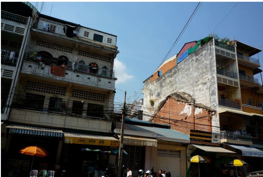
FIGURE 13: Evidence of demolished shophouses are often embedded like fossils on walls of neighboring buildings. The process of demolition and infill construction is how Phnom Penh has continuously regenerated itself.
