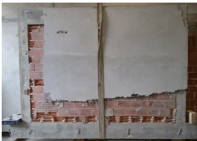
Figure 5.16 View of the crushing of bricks of the infill after removing some parts of the retrofitting layer in specimen SIF(CTRM)-I-2L(NC)-B
