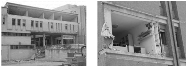
Figure 2.18 Damage in non-structural elements [19]
