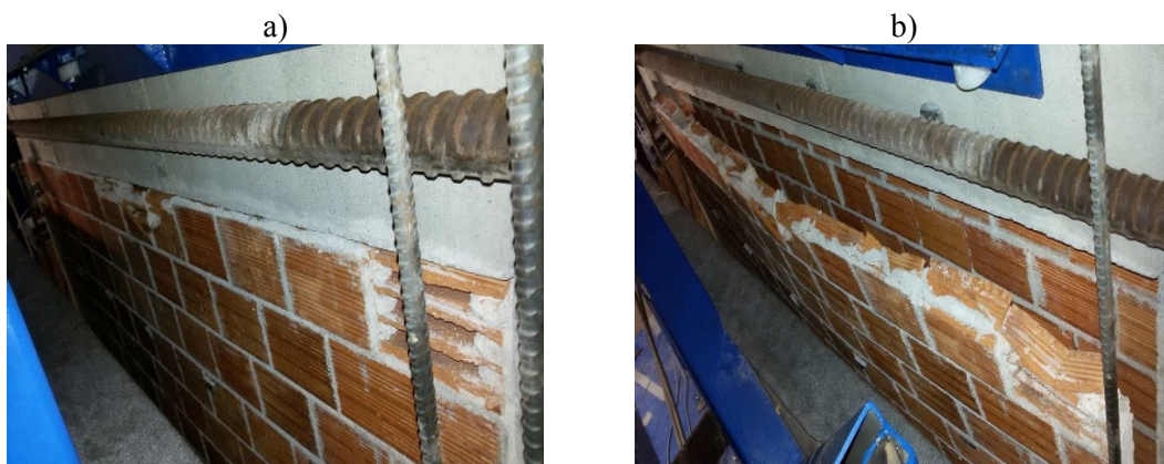
Figure 3.31 Out-of-plane bulging of the interior leaf during in-plane loading at lateral drift of a)1% b)2%
