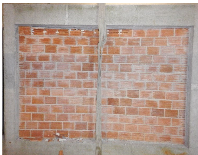
Figure 5.47 Out-of-plane damage in the interior part of the infill
