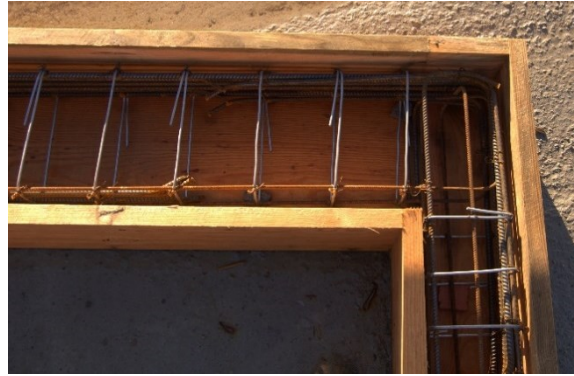
Figure 3.10 Absence of stirrups in the connection point of column to beam
