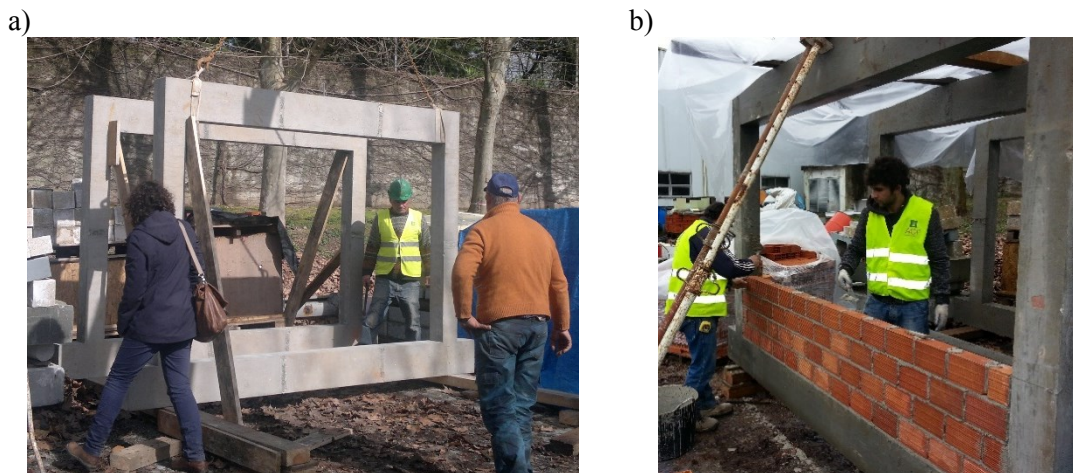
Figure 3.12 a) Transportation of the frames to the storage area and b) construction of the infills
