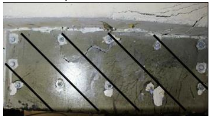
i) Crack pattern in the lateral surface of T-5L45-BC beam at failure load
