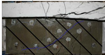
j) Crack pattern in the lateral surface of T-D-5L45-BC beam at failure load
