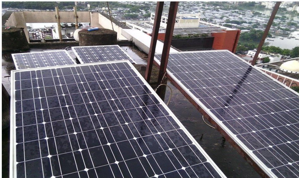
Fig 3.7: Solar Panels on the rooftop of BRAC University UB02
