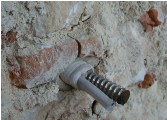
Fig. 6 Typical masonry failure mode during pull-out tests
