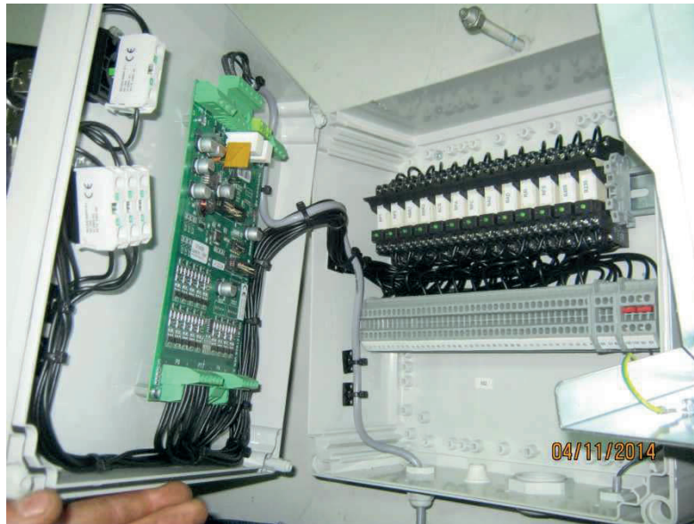
Figure 1 FEMS interface for Hydroware controllers
