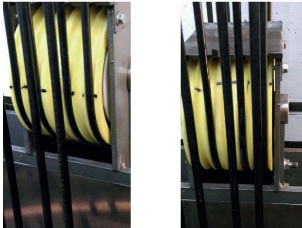
Figure 7 / 8: New solution before at installation / after 1 week operation
