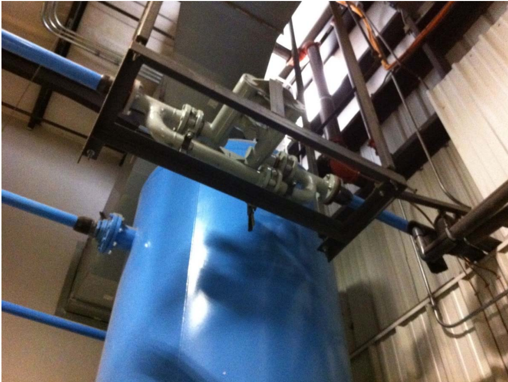
Figure 2-5: Pressure/flow controller regulating plant pressure to 85 psig. Bottom view with tank shown. Photograph by A.C. Harding, used with permission.
