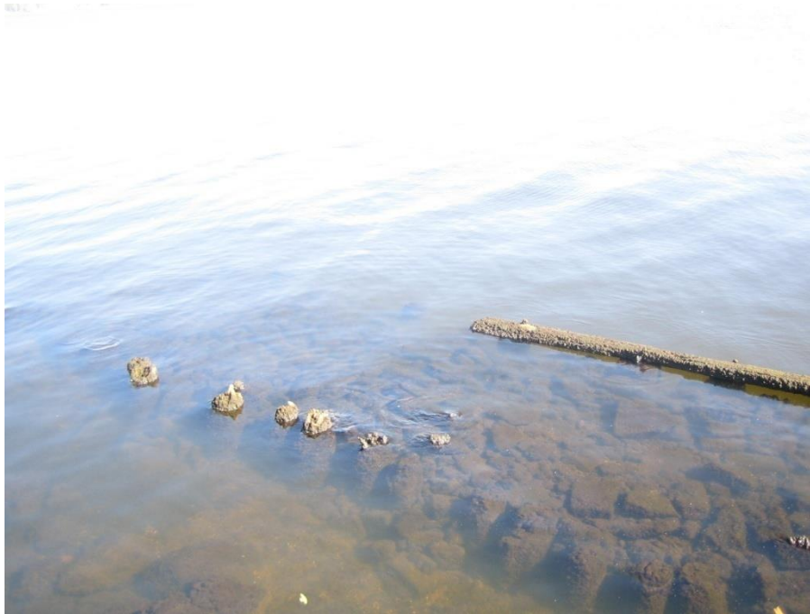
FIGURE 6.13. Photograph taken from Union Point Park, facing east. Pilings run parallel to the bank (Photo 23 taken 11/16/2007 by Jeremy Eamick).
